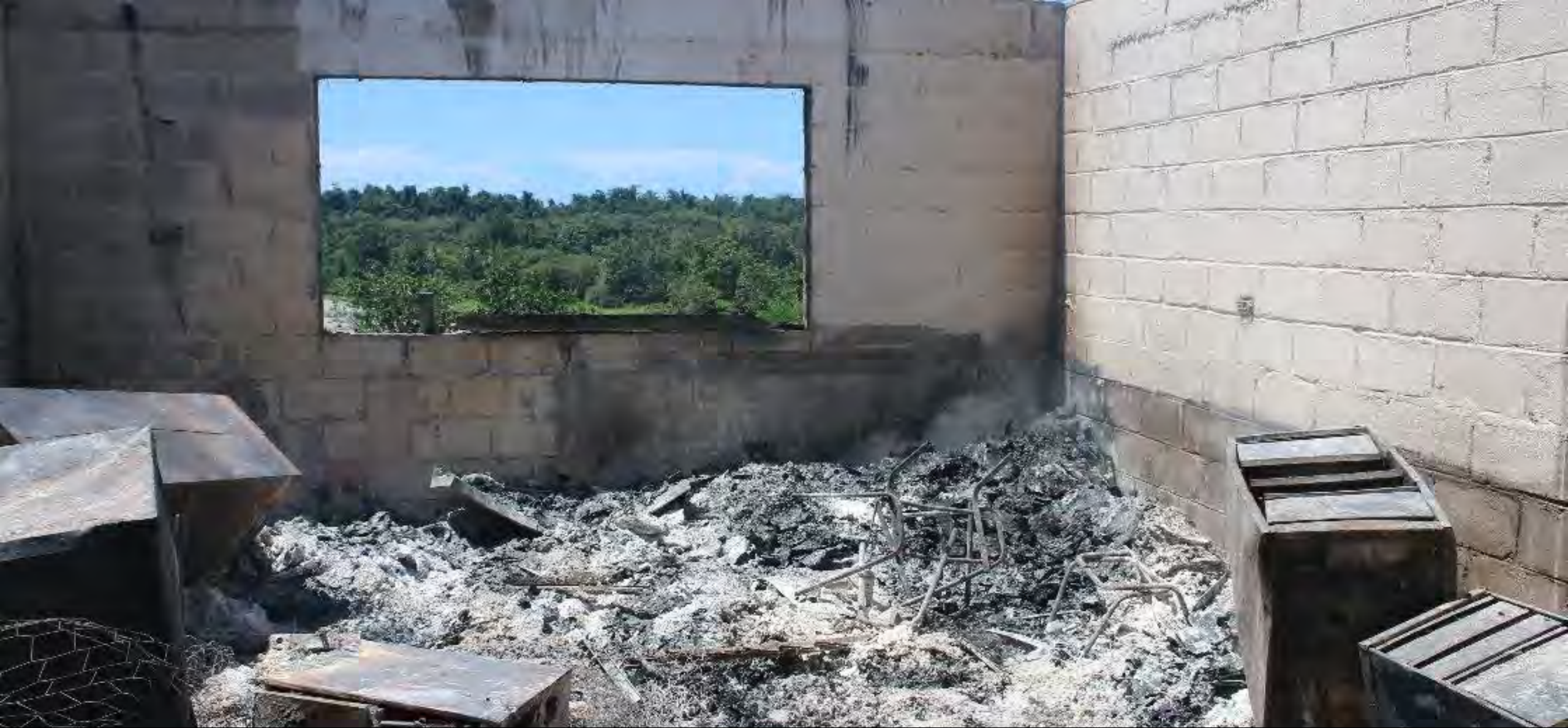
Remains of cabinets in the Students resource centre. This room stores all students text books and other materials.
