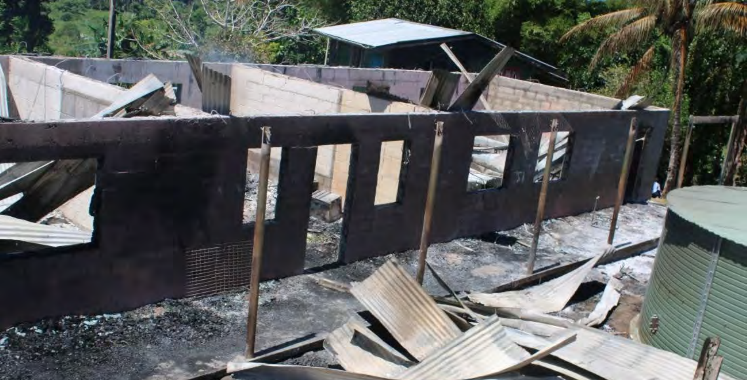
Aerial view of the burnt classroom block.
