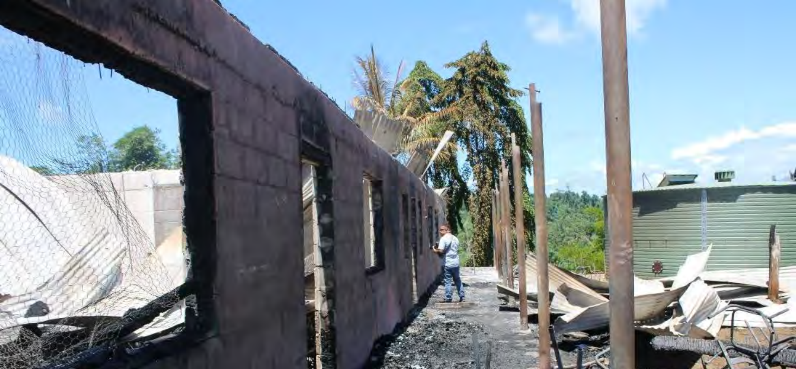
Front view bottom floor of the two-story classroom block that burned.
