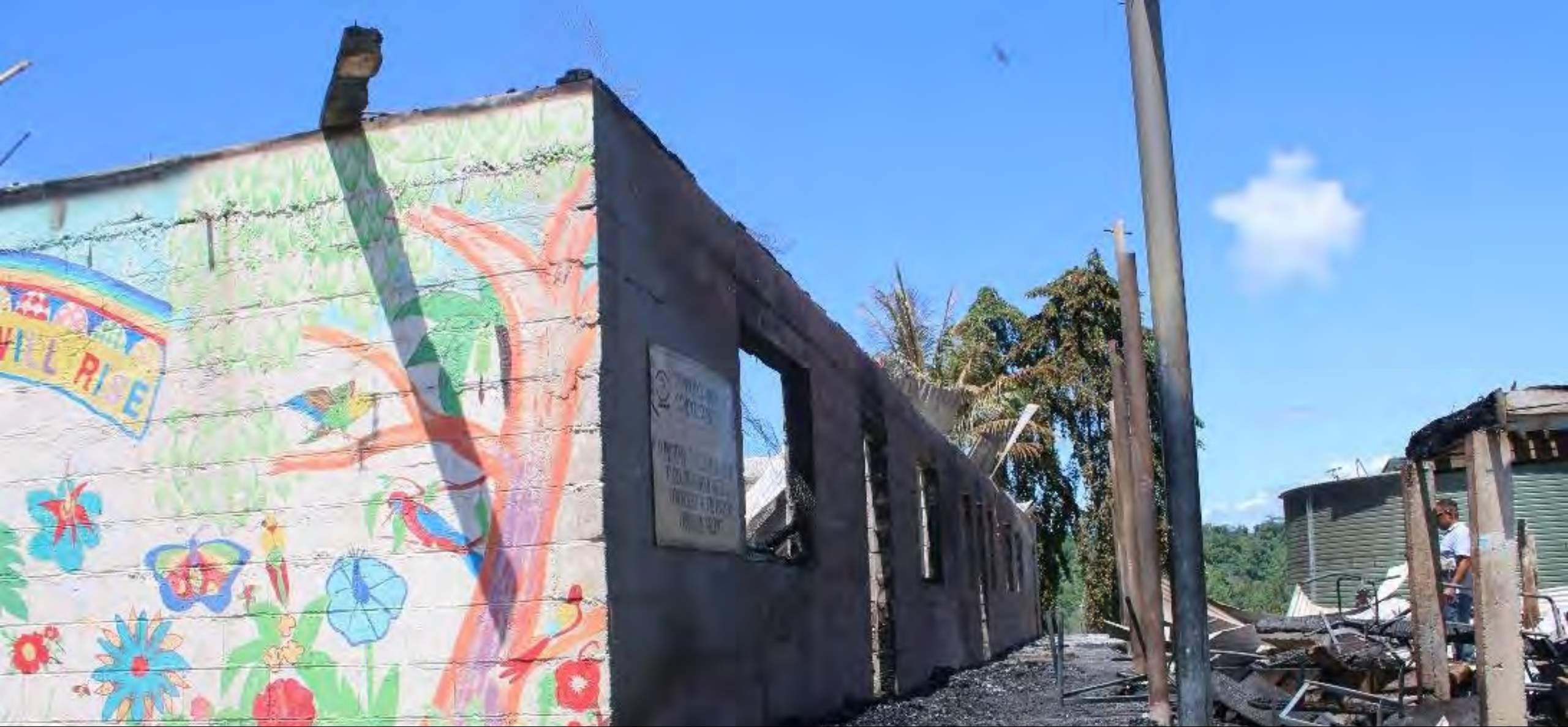
Front-side view of the remains of two-story classroom block that burned.
