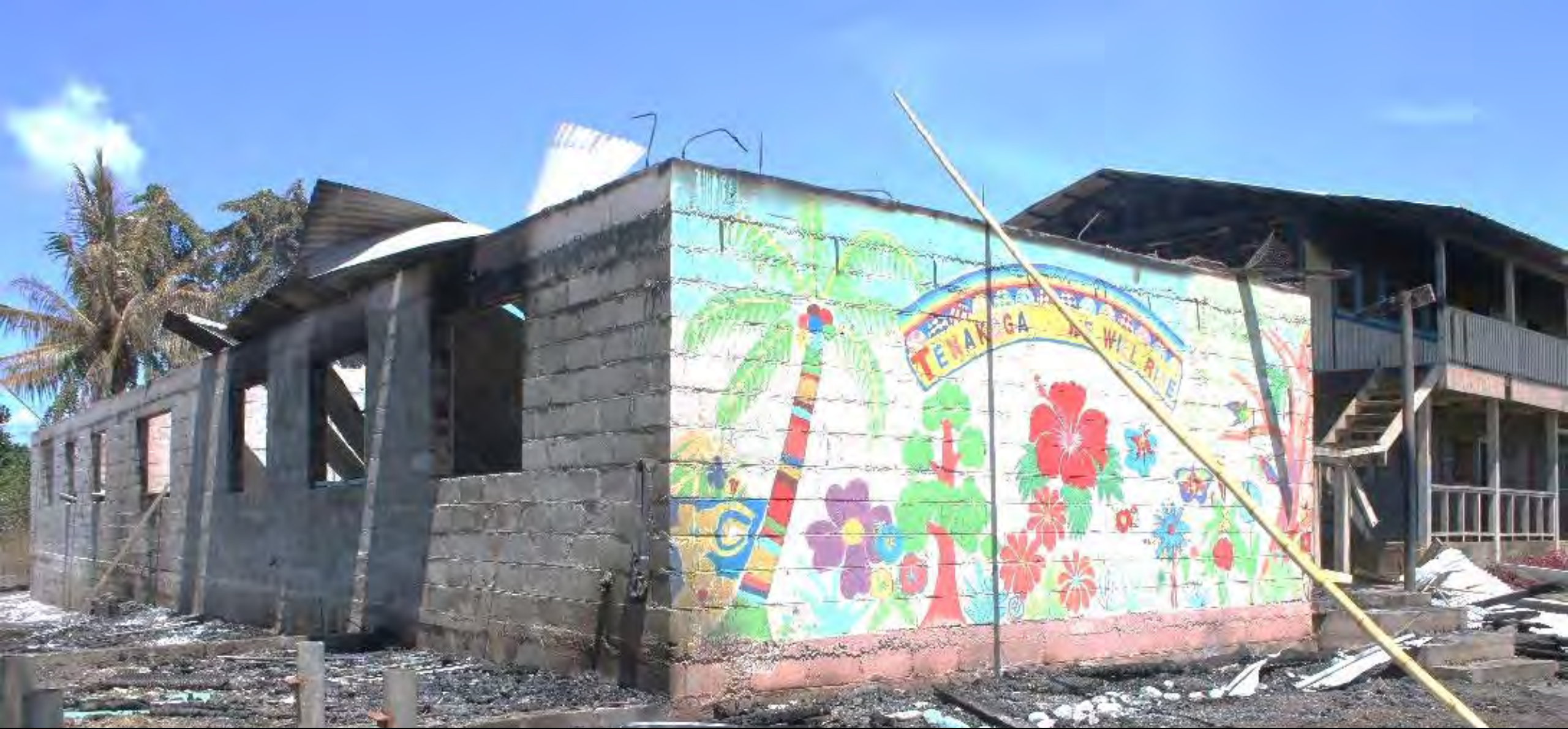
Back-side view of the remains of two-story classroom block that burned.
